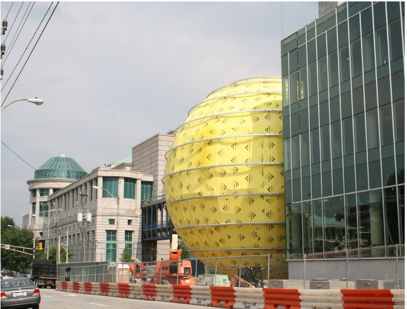
Construction of the SECU Daily Planet in August 2011 on Jones Street, Raleigh, NC.
